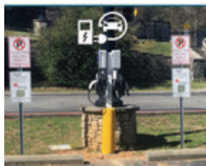
Free EV Charging Stations on Planer Hill at Transit Station.
